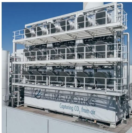
Figure 9. Large-scale installation of DAC in Switzerland.
