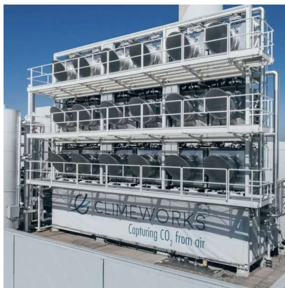
Figure 9. Large-scale installation of DAC in Switzerland.
